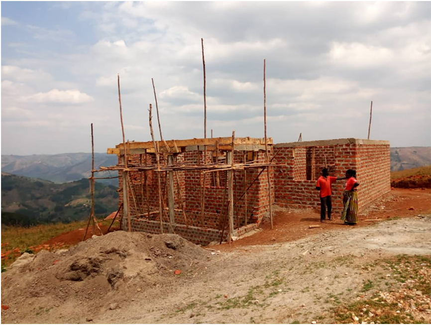
Figure 1. A small, half-built, brick house on the outskirts of Mbarara. This modest construction project was already two years in the making when this photo was taken. Photo by Twesigye Pius.
