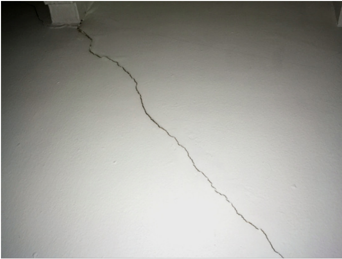
Figure 9. The beam where Elena thinks her apartment's crack emerged. Photo by Lachlan Summers.
