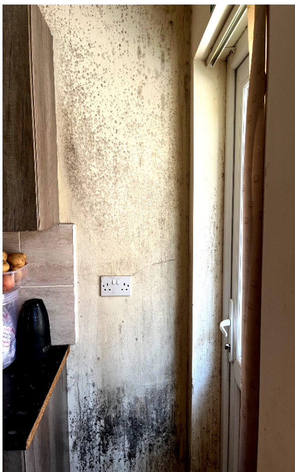
Figure 4. Mold growing in the kitchen of a council-owned temporary accommodation house inhabited by a Somali woman and her family.
