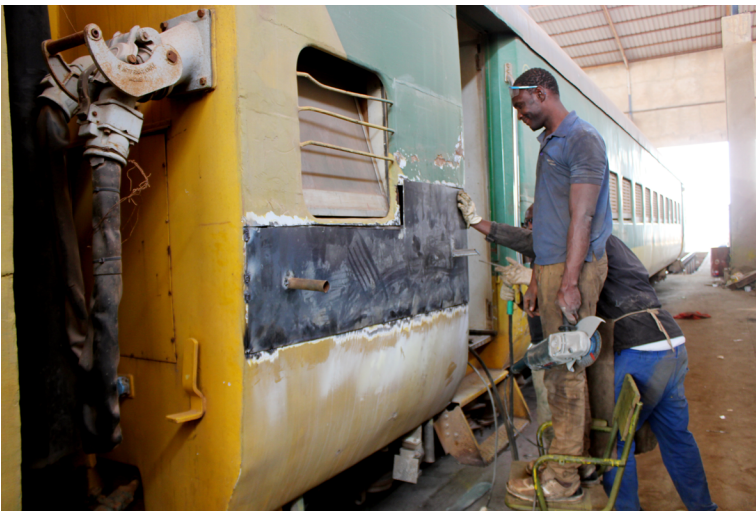
Figure 3. Surface repair on a passenger carriage in the Rufisque workshop that improves the exterior while leaving mechanical issues untouched. Photo by Charline Kopf.
