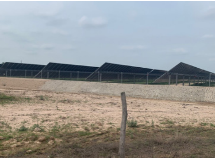
Figure 6. La Loma Solar Park. Photo by Juan Pablo Vera Lugo.
