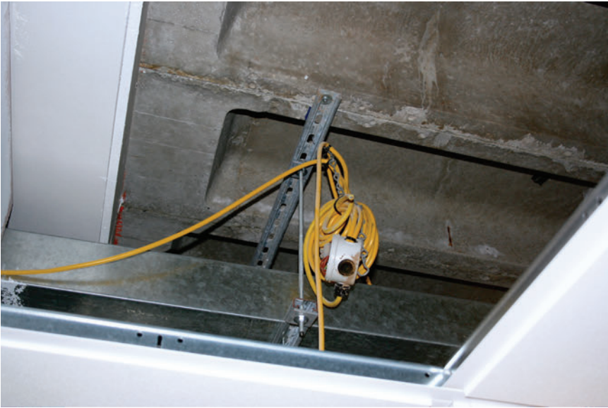
Figure 3. Here, in a modern office environment, lines of electrical conductivity are hidden in an overhead void. We only catch sight of such lines when maintenance is needed, briefly revealing a world of threaded currents. Photo by Mike Anusas.
