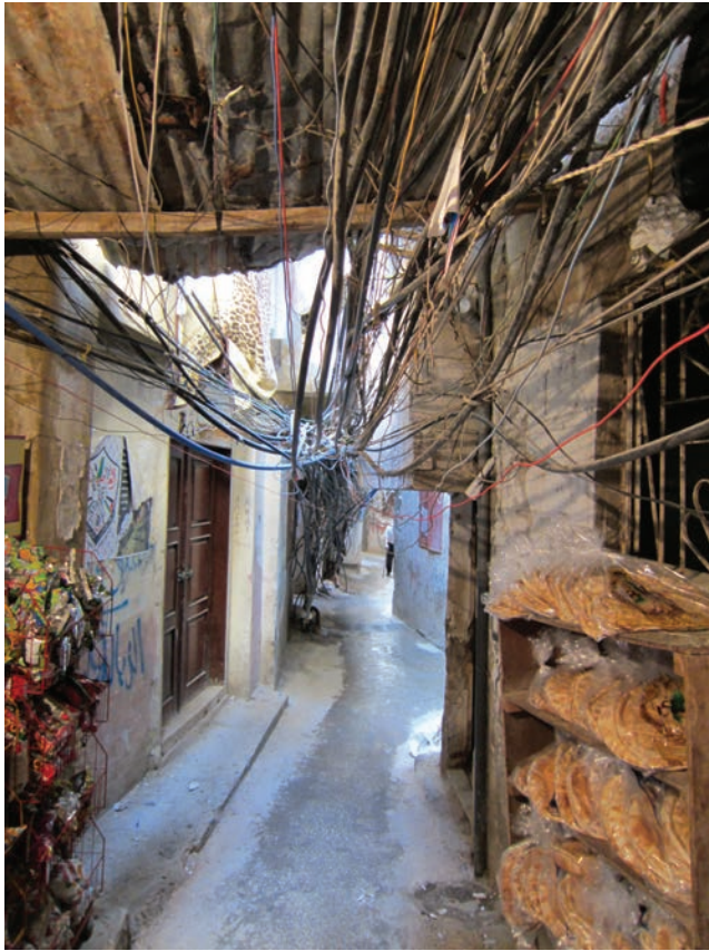
Figure 3. Electric wires over a camp street. Photo by Ilana Feldman.
